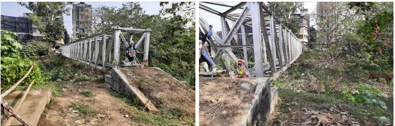
Arrangement to Avoid Interference with Drainage in Kamakhya – Paltanbazar 132 kV UG Cable
