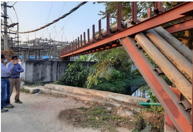
33/11 kV Ulubari Substation (Existing)
